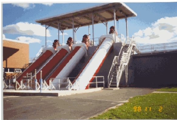
Screw Pumps lift the water from the Primary clarifiers up into the aeration/nitrification tanks. Each screw pump can move 7,600 gallons per minute.
